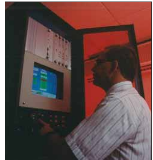
Touch screen monitor is a user-friendly way to supervise RF links and remote station status.
